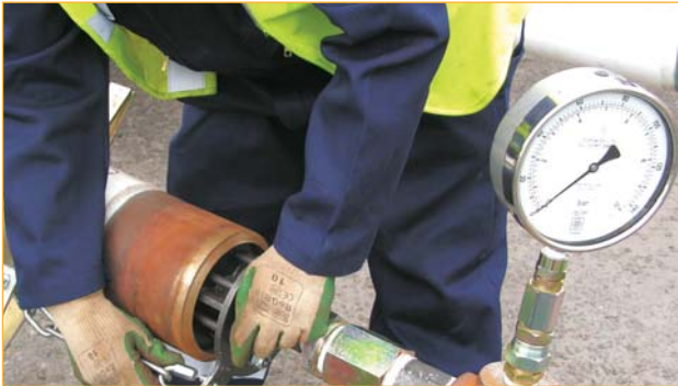
A pressure of between 8 - 14 PSI was applied to the PIG as it was launched down the pipe
