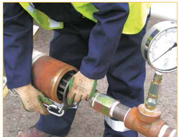
Air pressure being applied at the launcher
